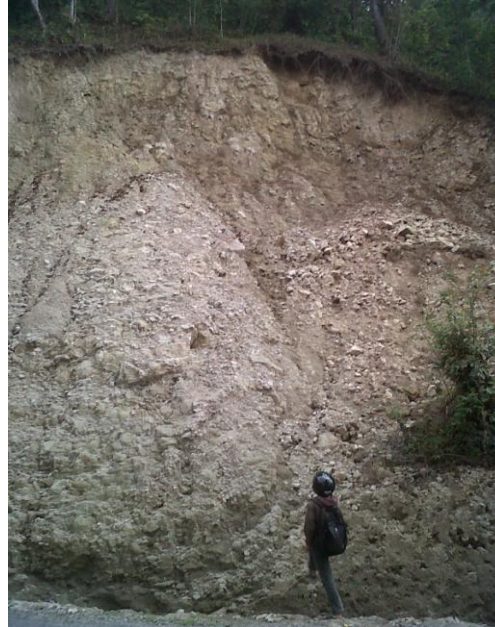
Figure 6. Landslide due to Cutting Slope for Road
